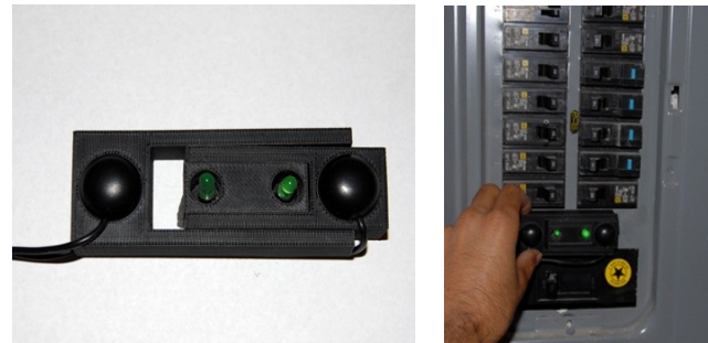
Figure 1: Left: Contactless, whole house power consumption sensor. The sensor can be adjusted to accommodate most electrical breaker panels. Right: Sensor installed on the outside of the breaker panel.
